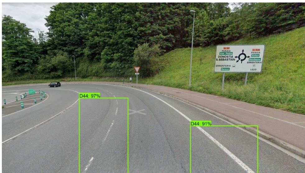
Figure 5-6. Road marking damage detected in GI-636 exit branch road.
